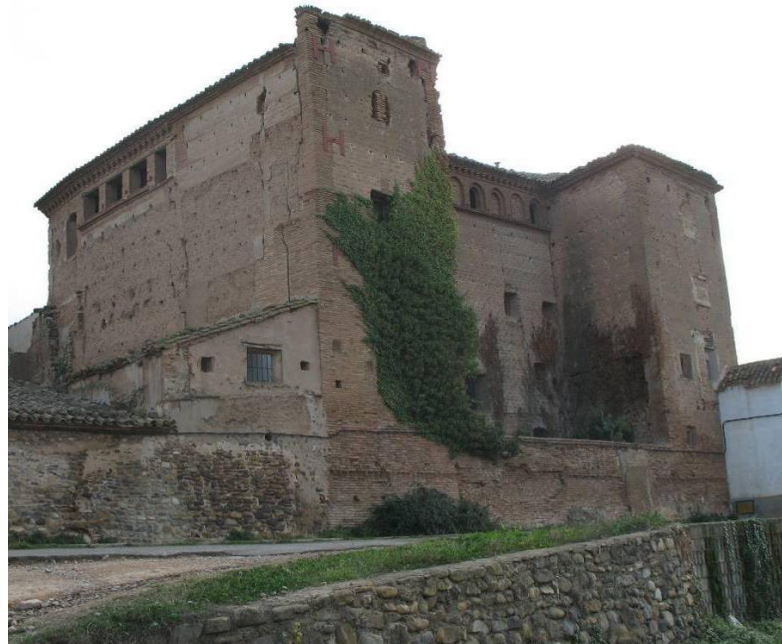
Figure 1 The preceptory at Ambel, north-east elevation. The gallery of arches between the towers is typical of 16 th century architecture in this region. The first phase precinct wall reaches the base of ivy and stands 3m high.
