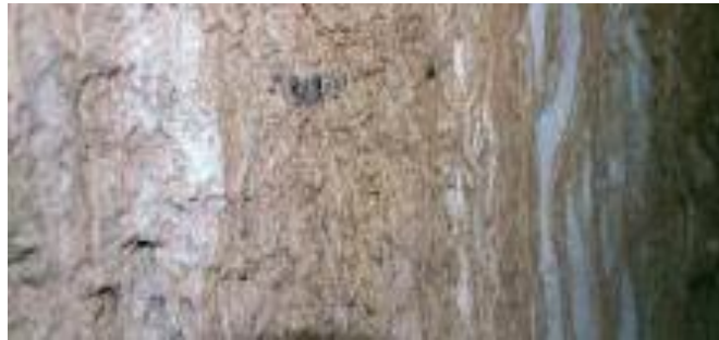
Figure 5 Worm cast type structures visible at Ambel beneath a previously damaged roof section
