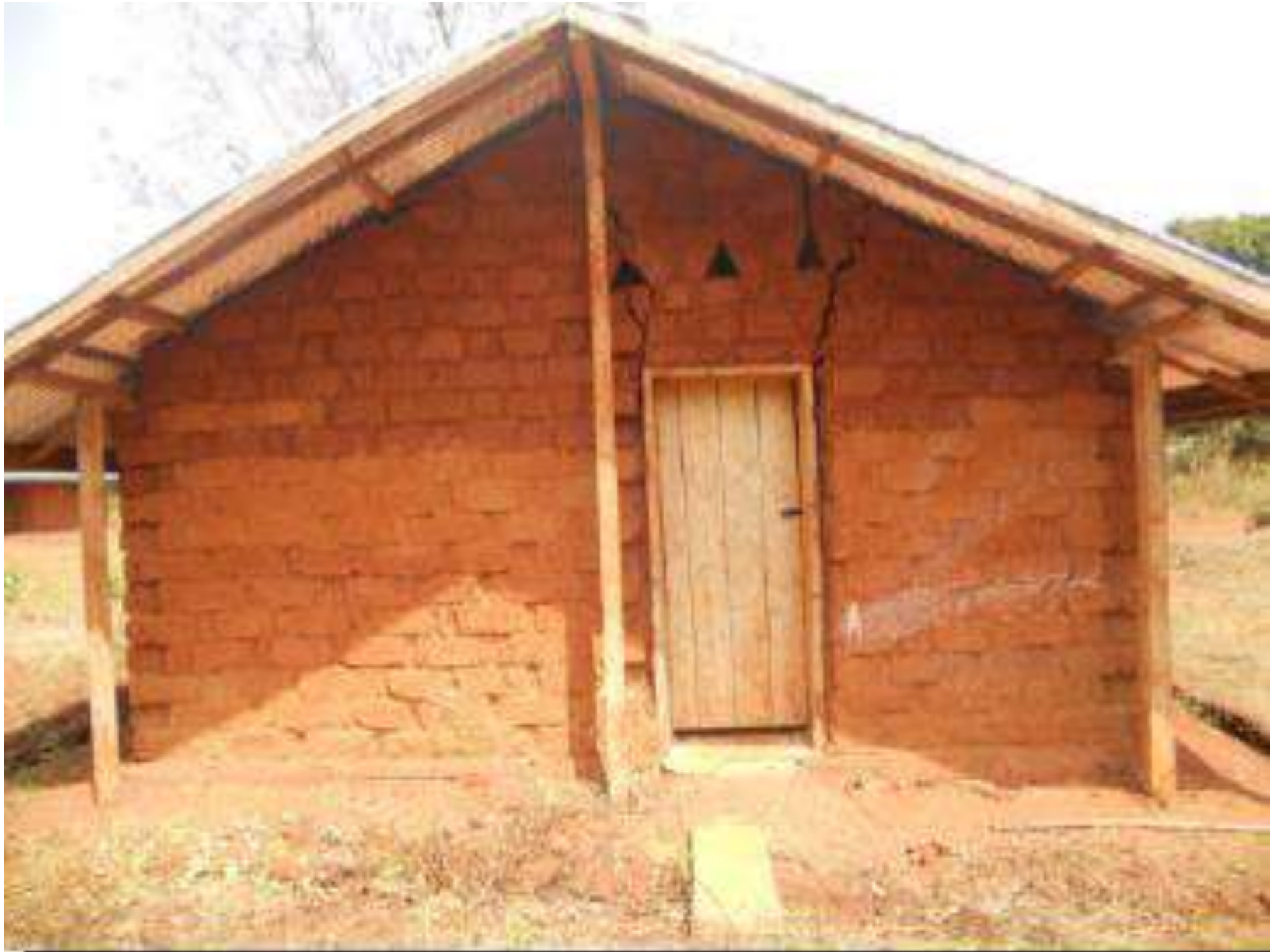
Poor design and construction happens without good guidance
